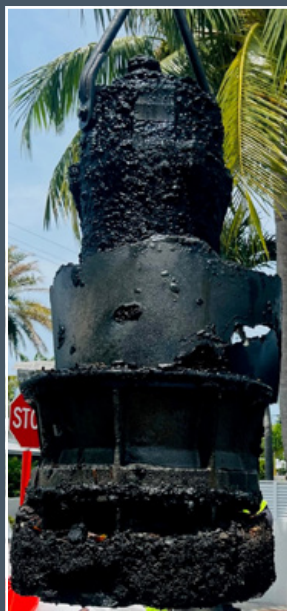
CAST IRON - 3 Years: Required Replacement
